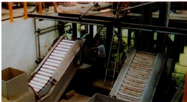
▲ Line and automated knock-out
