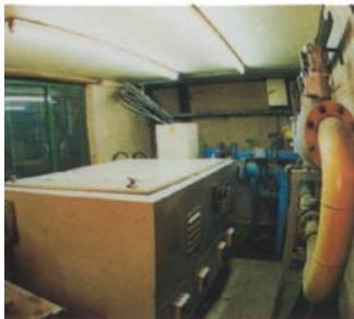
▲ Mains power transformer
